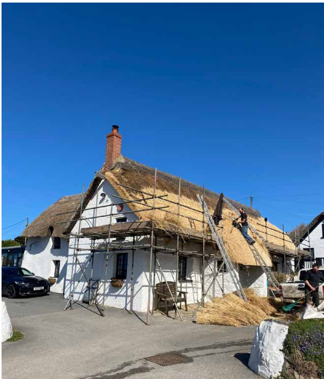
Figure 6 Grade II listed Treguth Inn, an early 17th century former farmhouse. Traditional materials include rendered and painted slate rubble and cob with a thatched roof. The intricate roof form is varied with both gable and half-hipped ends, and photographed being maintained through traditional methods.
